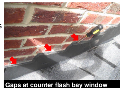
Gaps at counter flash bay window
