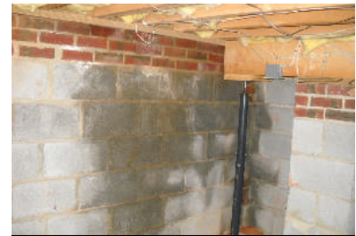
Wet walls at front by porch
