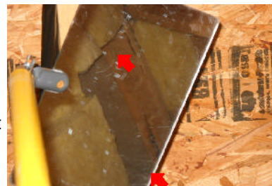
Missing insulation top of master bath
