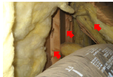
Missing/fallen around master bath
