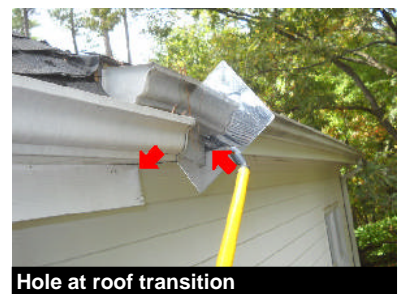
Rotted fascia at false gable/garage
