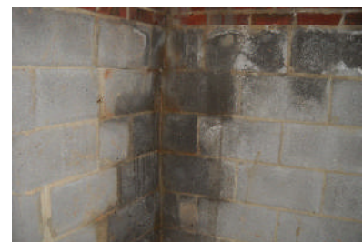
Wet walls corner right of porch
