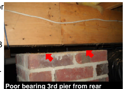
Poor bearing 3rd pier from rear
