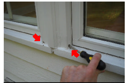
Several rotted areas/sunroom wind.
