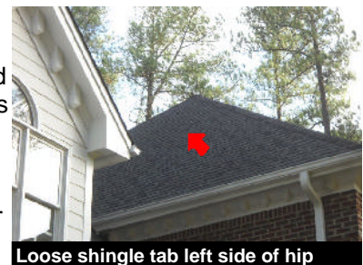
Loose shingle tab left side of hip
