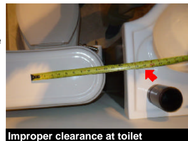
Improper clearance at toilet
