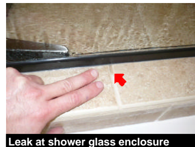
Leak at shower glass enclosure
