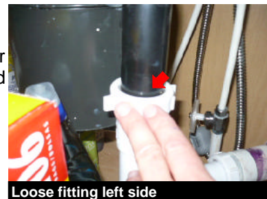
Loose fitting left side
