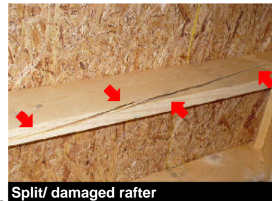
Split/ damaged rafter
