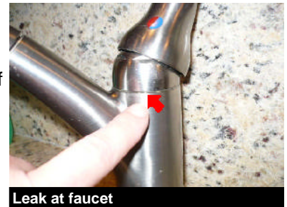
Leak at faucet
