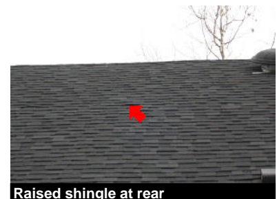
Raised shingle at rear
