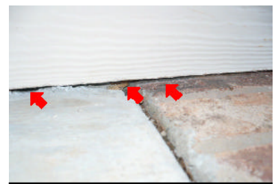
Caulking needed at siding and porch
