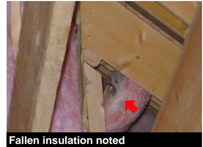
Fallen insulation noted
